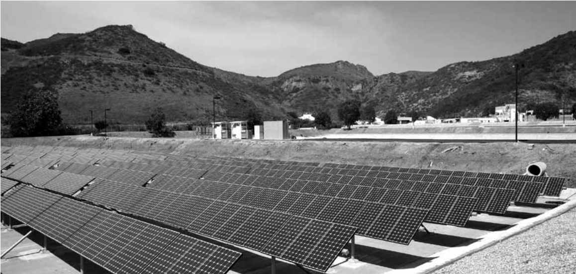
Solar Array at the Hill Canyon Wastewater Treatment Plant, Camarillo, California. The Array provides about 15% of the facility's energy needs. PHOTO CREDIT: PETER BENNETT/GREEN STOCK PHOTOS
