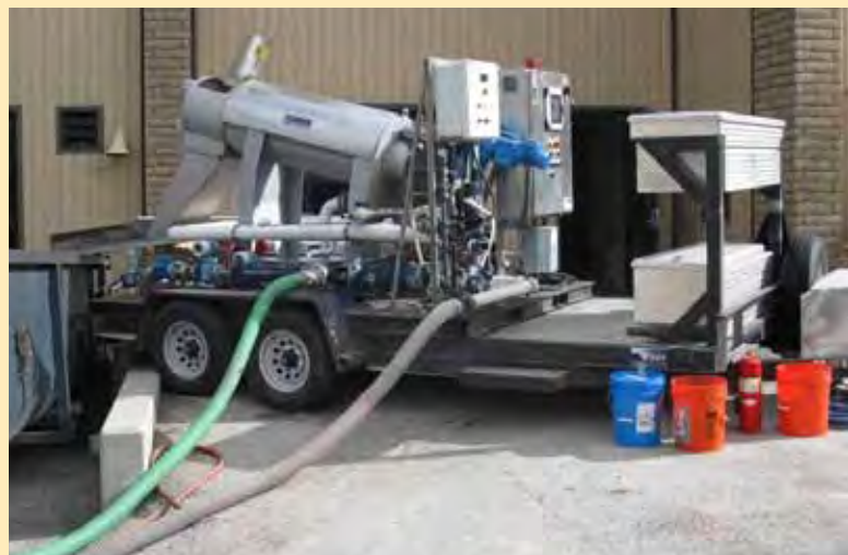
SCREW PRESS AT THE SALMON CREEK WWTP
